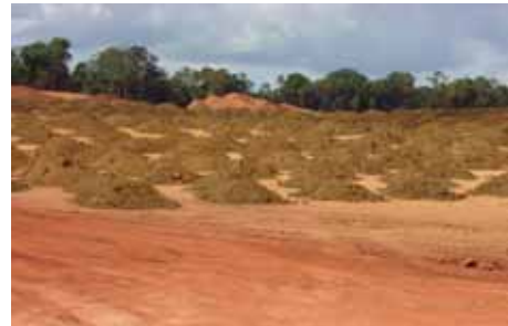
Figure 6: Stockpiled soil rich in organic matter is returned to the site before revegetation
